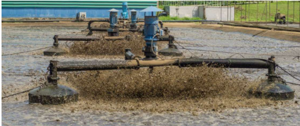
Activated sludge process
